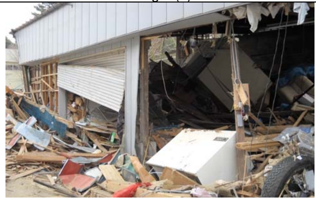
Photo 15: In the area where tsunami wave reached 1.8 m high, the first story was wrecked.
