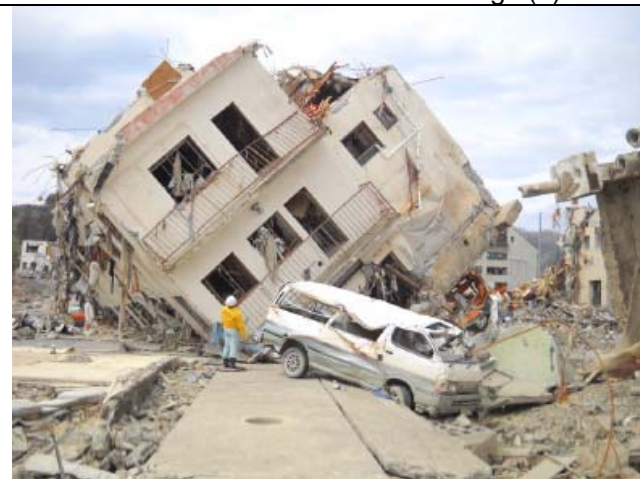
Photo 44: Overturned RC buildings (4).
