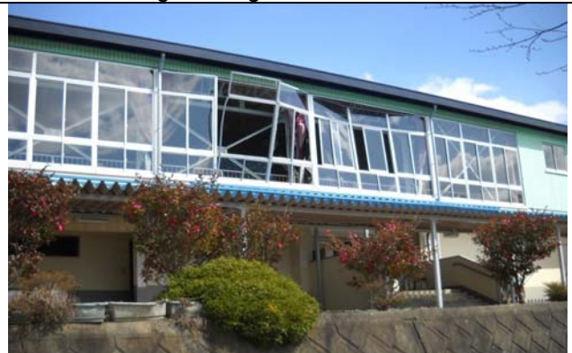
Photo 9: Window glasses were broken in the gymnasium (2).
