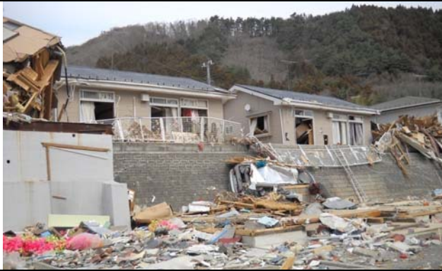
Photo 21: Total destruction of houses in low land (1).
